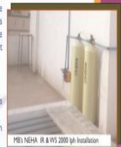
MB's NEHA IR & WS 2000 lph Installation
